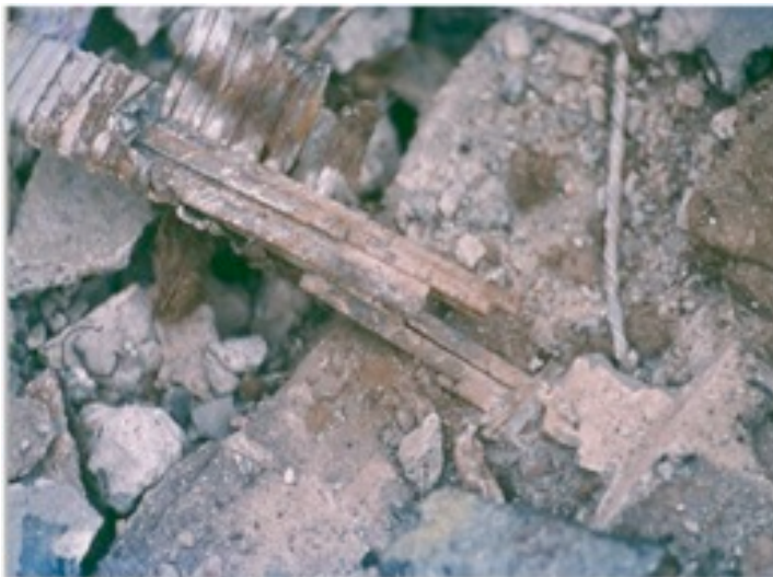
Cause of the collapse: stress corrosion cracking of prestressed steel in ring beam joint.
