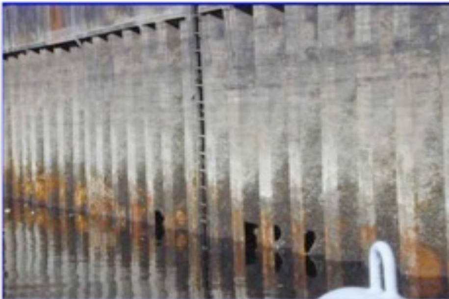
Figure 21: Low water zone corrosion of sheet pilings. 29
